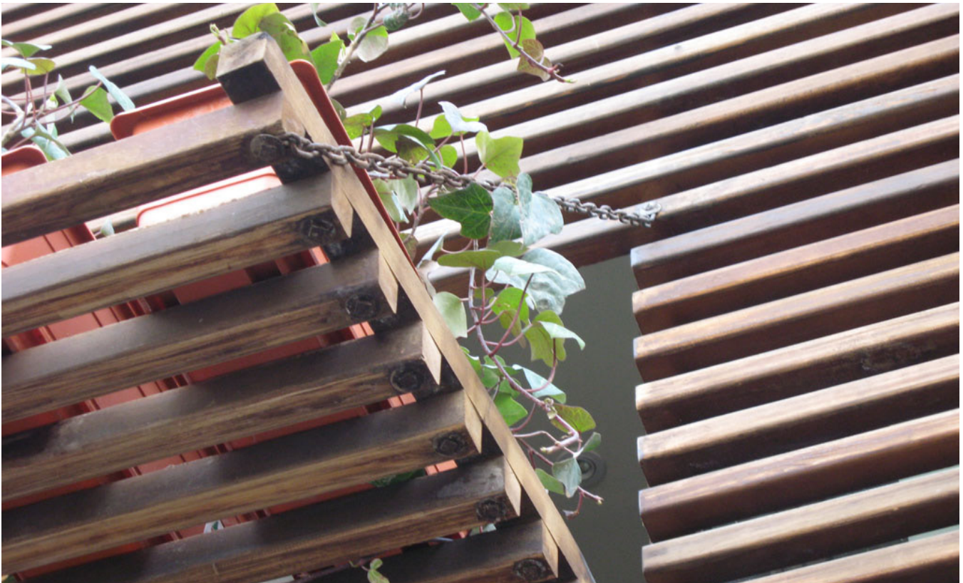
Detail of a panel with greens.
