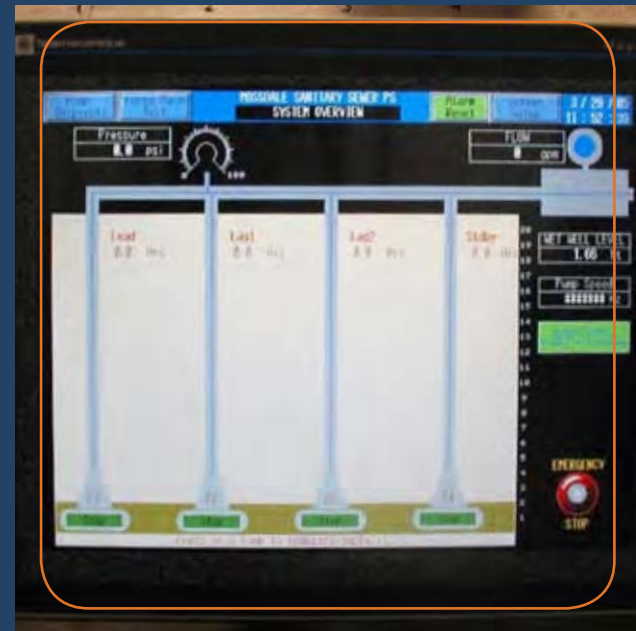
Local PLC Control System
