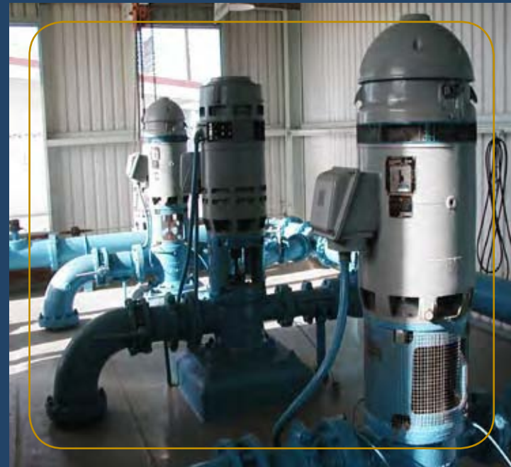
System Design Includes 2500, 1000, 500 and 200 GPM Flow Rate VFD Pumps Capability
