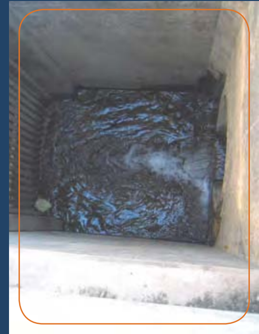
54" Stormwater Inlet Upstream of Screen in Low-flow Portion of Station (Main Station Filled Upon Overflow)
