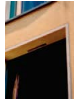
Air intake slit
