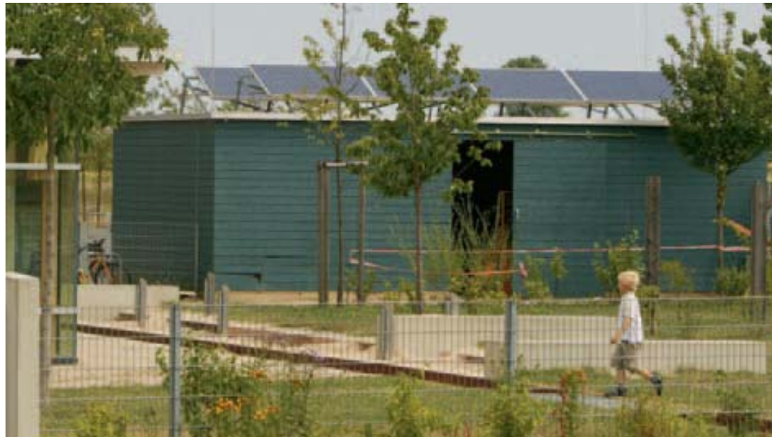
Photovoltaic installation at Kronsberg primary school
